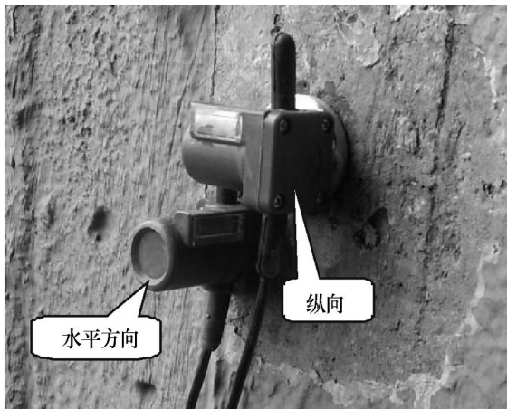
图 3 花果隧道左边墙测点照片 Fig 3 Point of measurement at left sidewall in Huaguo tunnel
